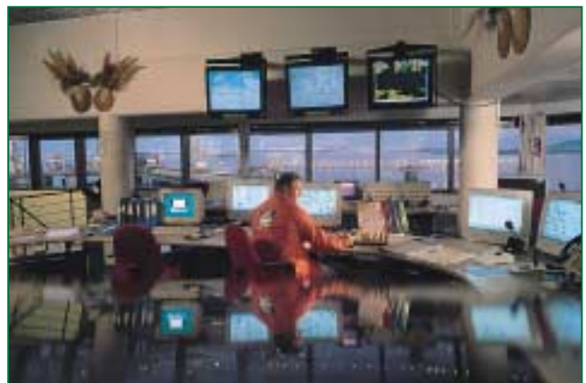
Scandinavian chic: the control room of the Sture oil terminal. ABB is modernizing the main control systems and integrating functions such as gas detection and emergency shutdown
